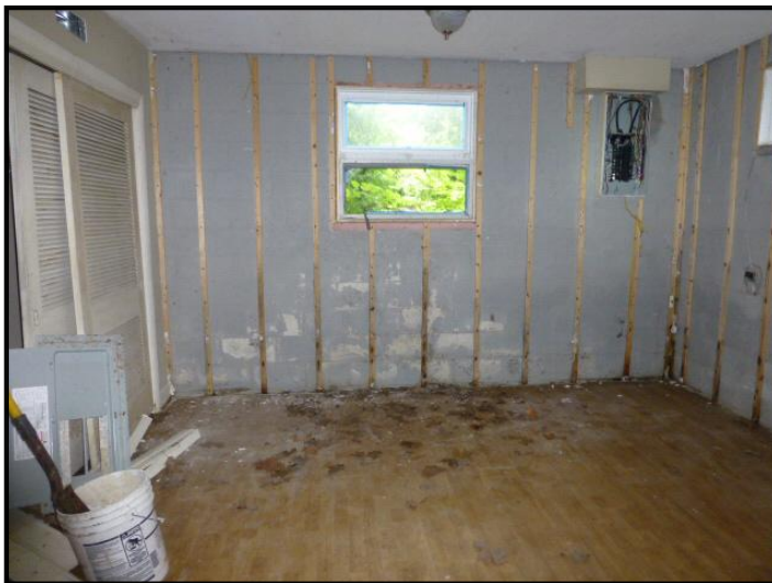
Moisture damaged bedroom walls removed on the lower level
