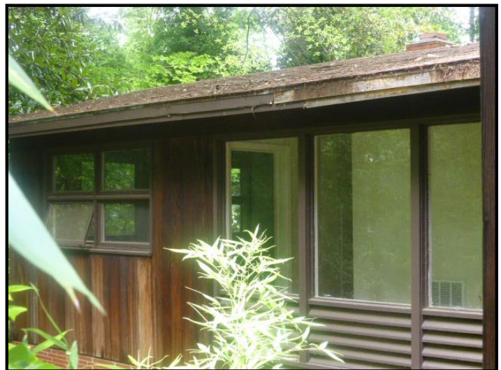
Damaged soffit/facia, and faded siding
