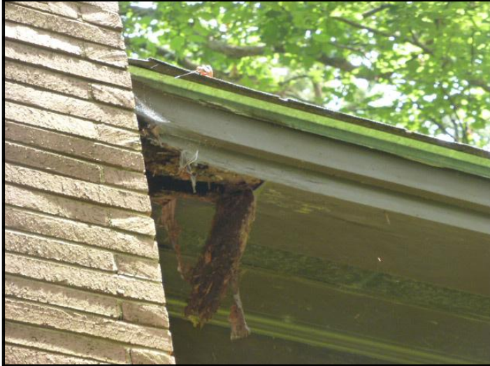
Moisture damaged soffit/facia
