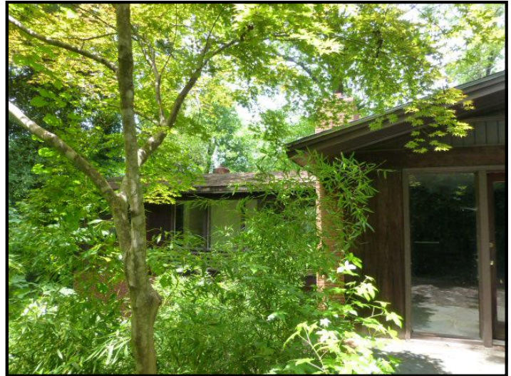
Steep drop off on left side of patio with no railing
