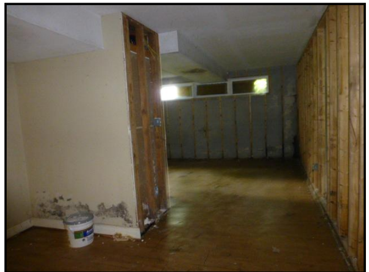
Lower level walls removed due to moisture penetration
