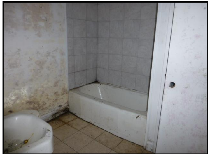
Lower level bath with moisture penetration to the outside wall
